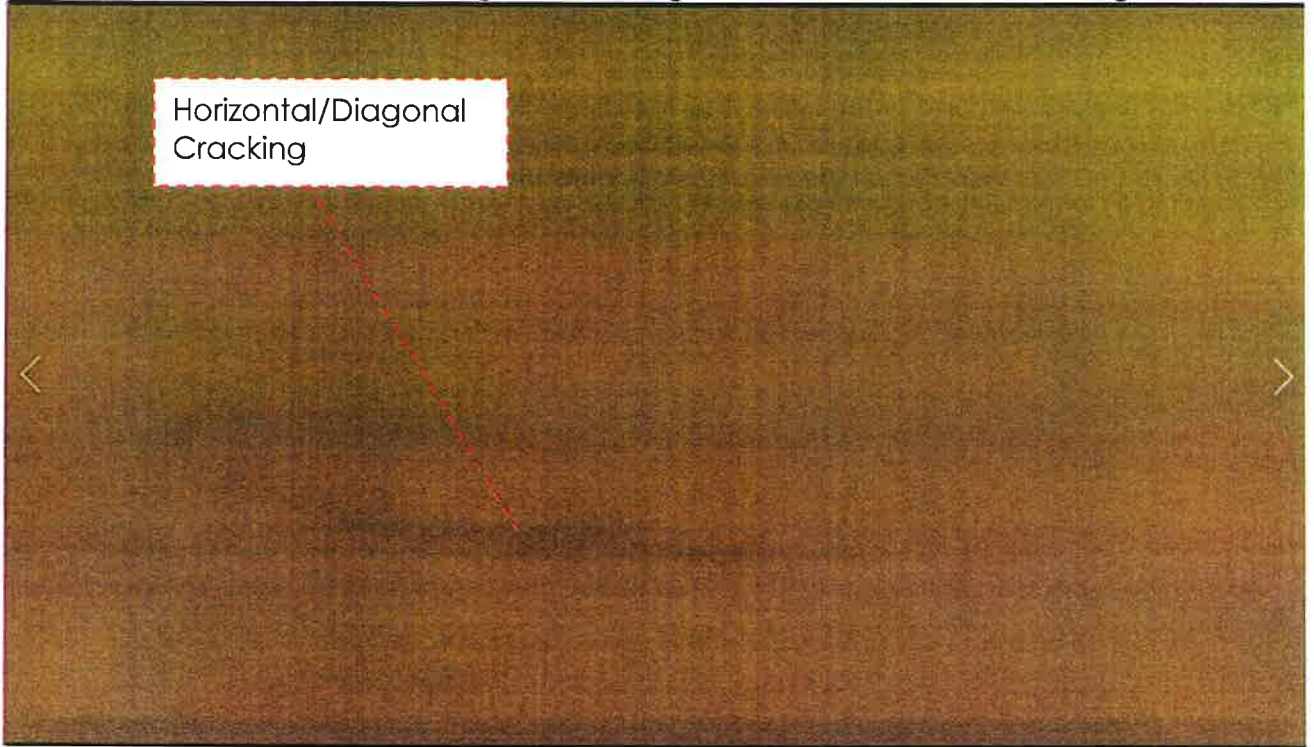
Photo #12- View of Horizontal/Diagonal Cracking in Slabs from Underwater Footage.
