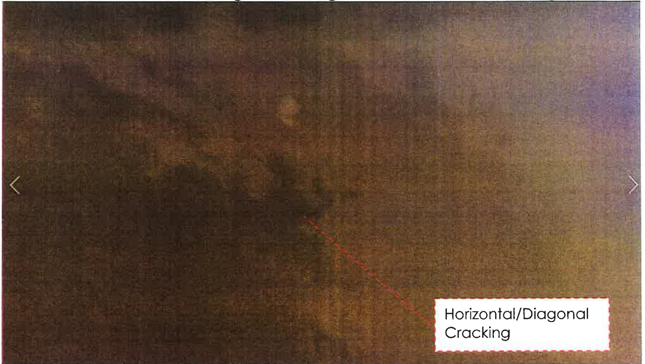
Photo #10- View of Horizontal/Diagonal Cracking in Slabs from Underwater Footage.
